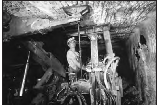
Installing roof bolts at a roof and pillar mining operation, Galatia Mine in southeastern Illinois.
